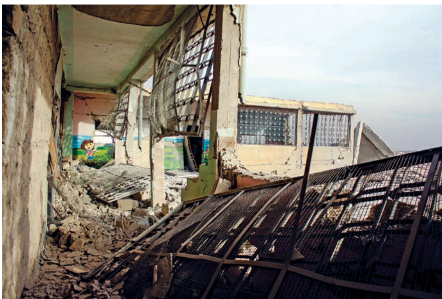
PHOTO: Russian airstrikes blasted open this school in Atarib, exposing the main corridor that led from the entrance to the classrooms. (SIJ)
